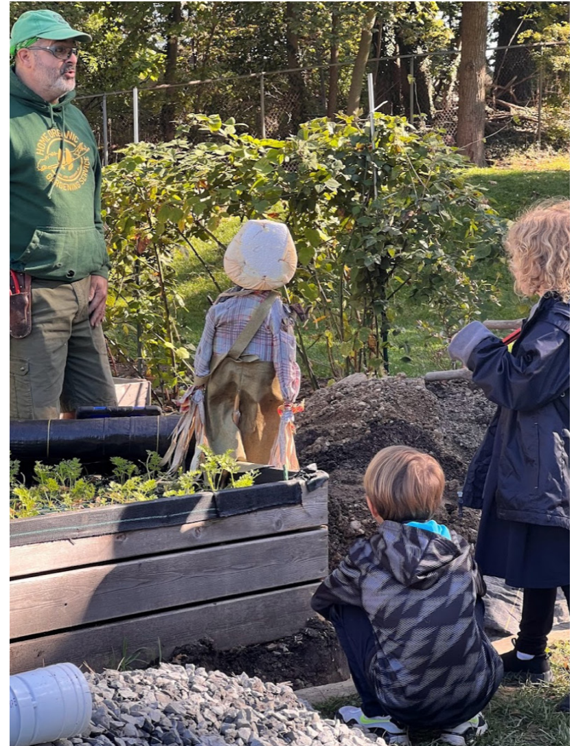
Learners help our Organic Gardening Specialist Mr. Dylan install french drains to save their Farm Stand crops from flooding.
